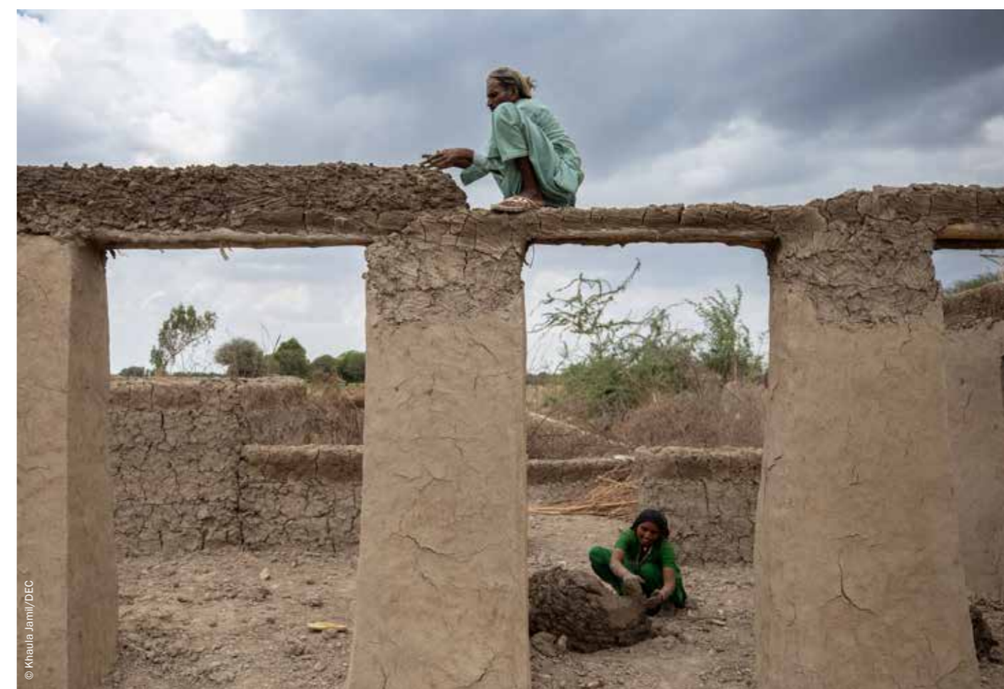
Village committee president and local farmer, Gulab and his daughter build a new mud house for their family. After the devastating floods in Pakistan, the local partner of a DEC member charity worked through village committees to help identify the needs of local communities and strengthen their capacity to achieve their priority goals.
