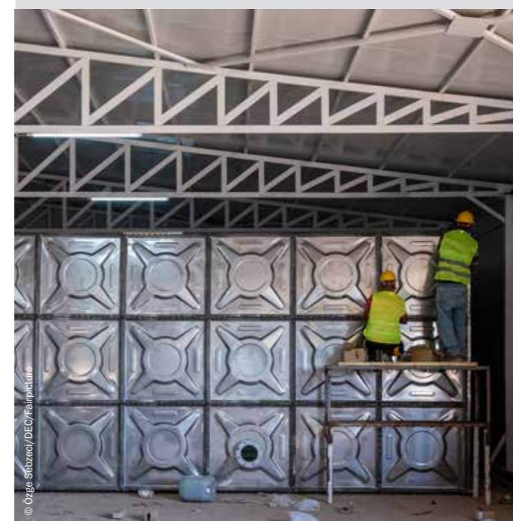
Construction work takes place on a large water tank in a container camp in Turkey, where DEC funds are supporting access to clean water for people who lost their homes in the earthquakes.
